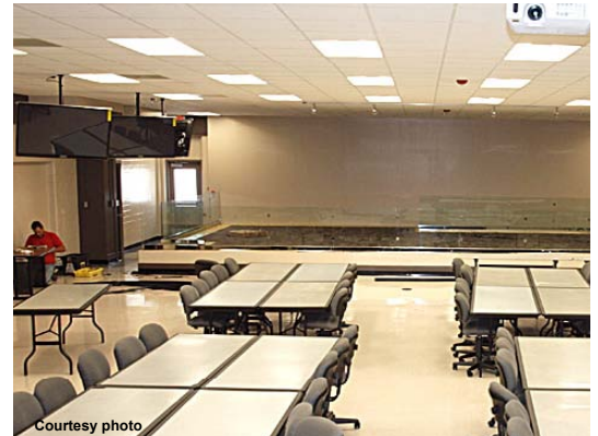
A contractor cuts the stage's rubber basing as part of the installation phase for its glass.
