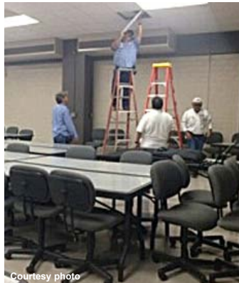
Following the installation of monitors, workers put the finishing touches on ceiling tiles.
