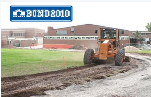
A road grader clears ground in preparation of a new all-weather athletic track at Edison HS. Cinder tracks at all eight of SAISD's high schools are being replaced.
