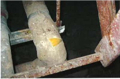
2. White Pipe Mastic – 4% Chrysotile Above ceilings, behind walls, mechanical rooms, and crawlspace
